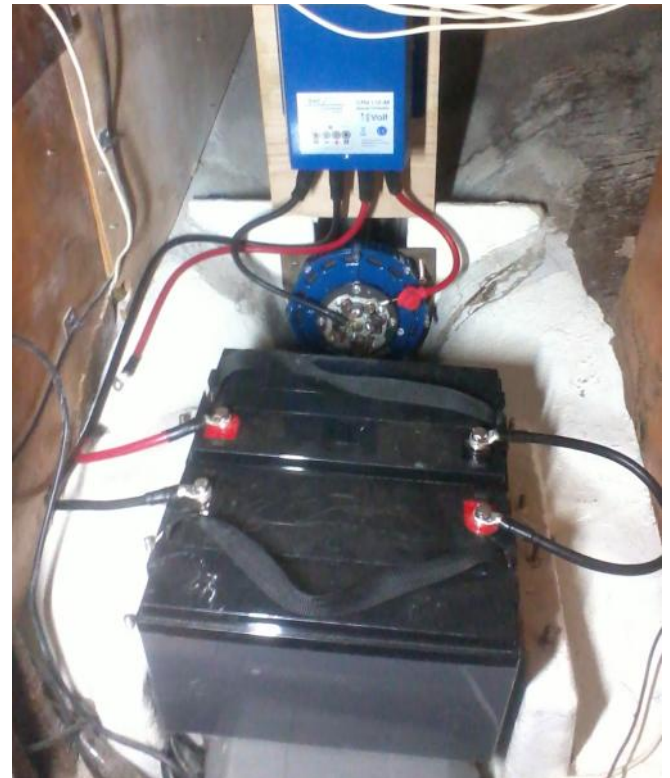
Controller, motor and battery bank
